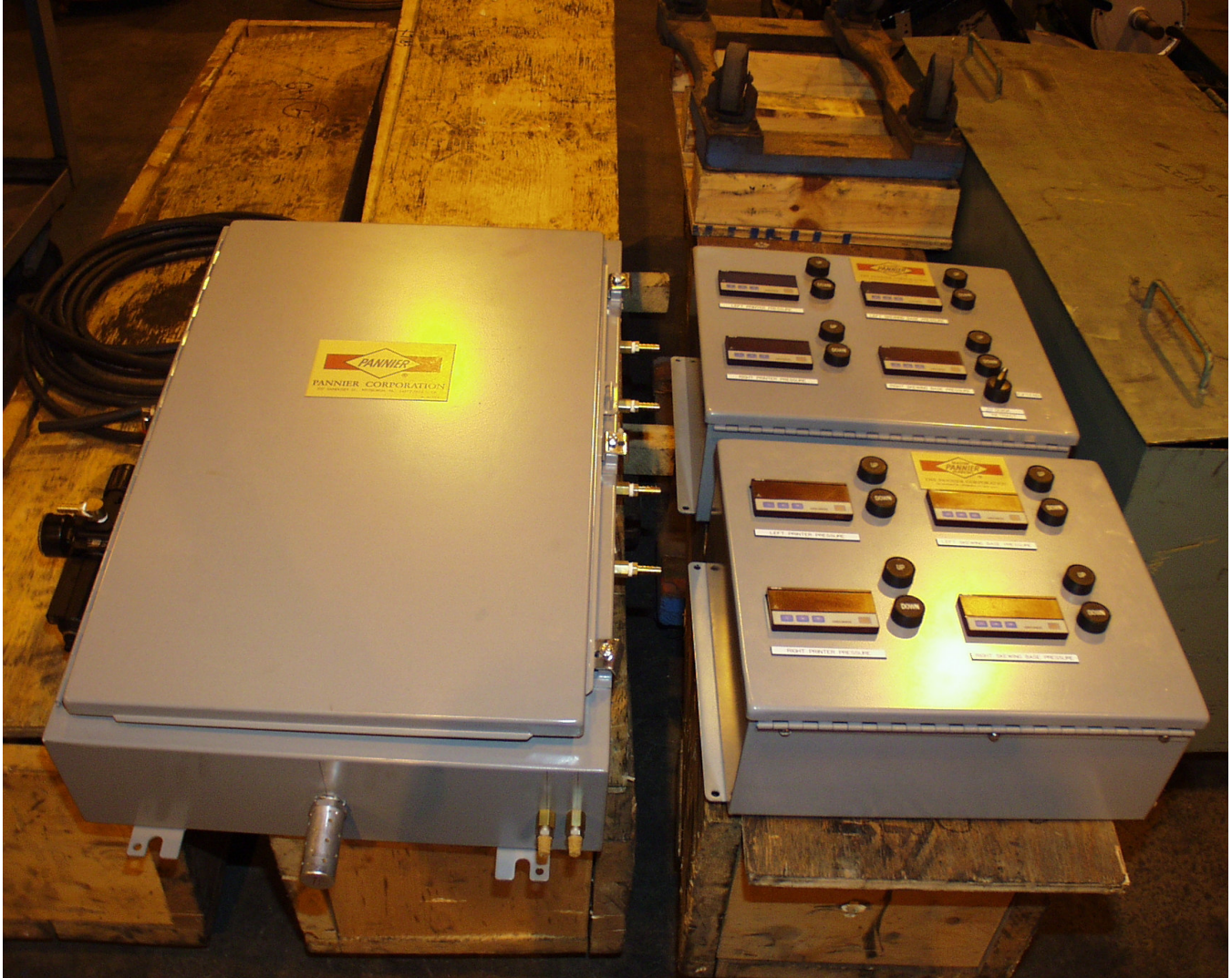
RPS Central Control Box with Pressure Control Valves and Two Control Panels
